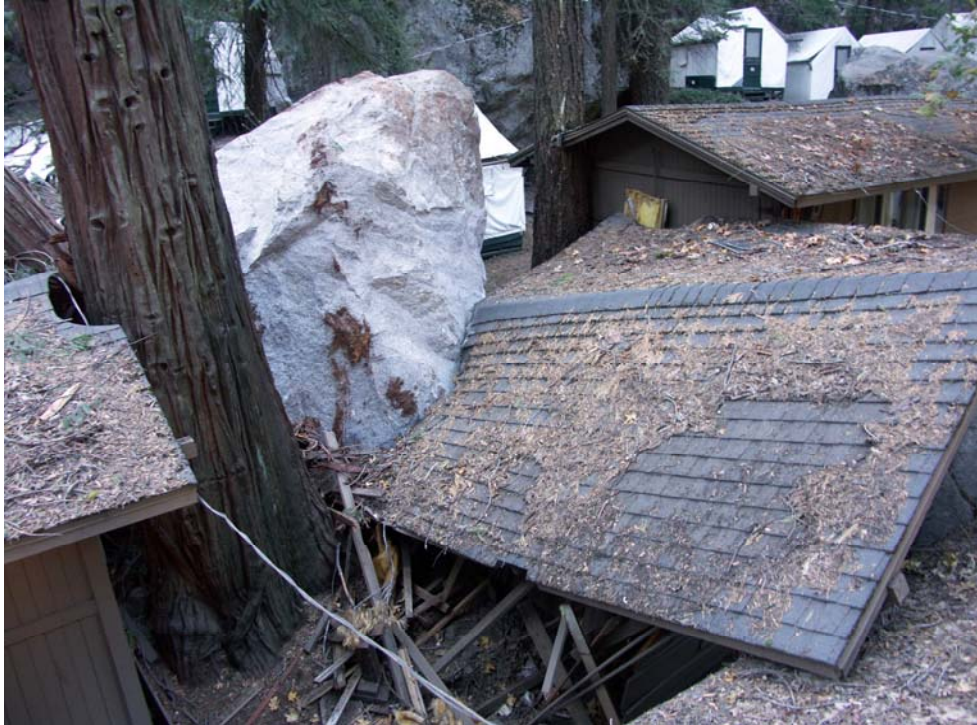
Figure 5. Cabin damage in Curry Village from a fresh, light-colored boulder resulting from the 8 October 2008 rock fall from Glacier Point. Darker-colored prehistoric rock-fall boulders can be seen in the background. Buildings in this region were permanently closed following the rock fall.
