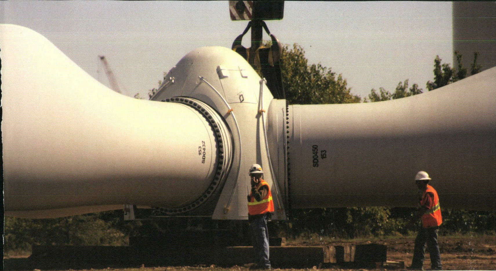
Two cranes were used to guide the massive turbines into place at Flat Water Wind Farm.
