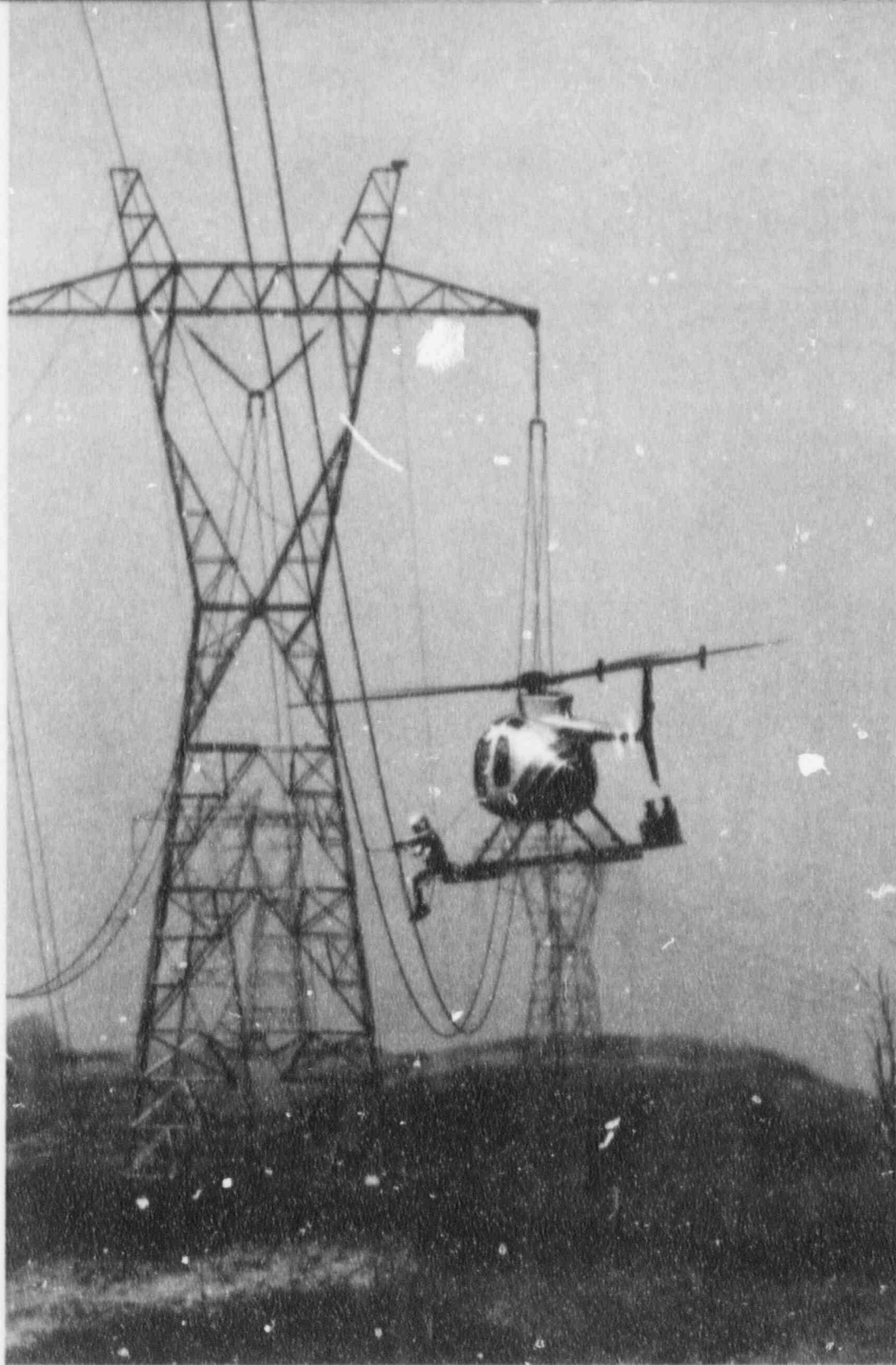
Using helicopters is an effective way to help inspect and maintain our 4,500 miles of transmission lines.
