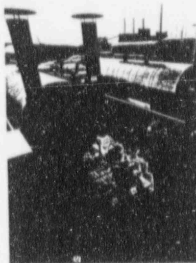
Oscar Langlois, watch engineer, supervises the monitoring of the pressure and temperature of pipeline gas that fuels Brayton Point Unit 4.
