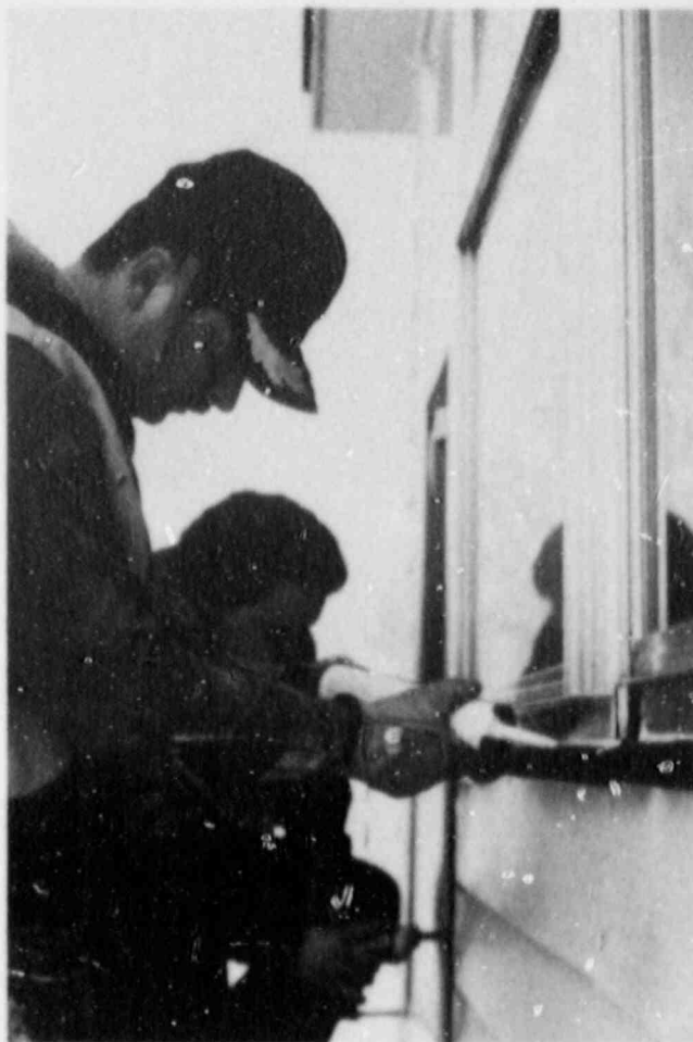
Jeff Morgan, left and Craig Scroggins from the Bethalto Jaycees caulked windows at the home of a widow. This was funded with a part of a $23,000 grant from the Energy Assistance Foundation. The Jaycees completed their three-year project in September 1987, weatherizing 34 homes.
