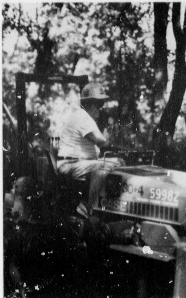
Main and service labor foreman Ralph Ohl helped dig a trench across the Kaskaskia river bed and through adjacent woods so the Company could begin supplying natural gas to a subdivision near Carlyle.
