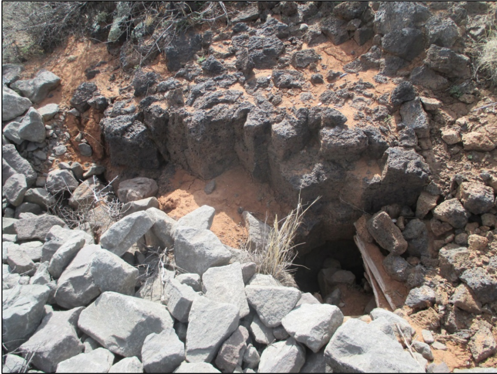
PL-17. Settlement in Fill Covering Basalt at the Interface of the East Dump Cover
