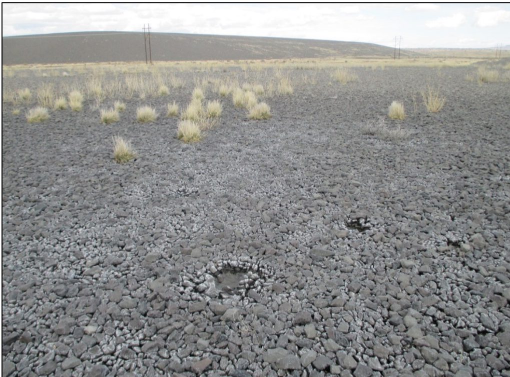
PL-12. Minor Ponding in the Shallow Depression on the Northwest Extension of the Carbonate Tailings Disposal Cell
