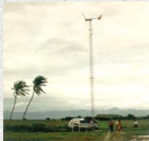
10-kW turbine directly coupled to a water pumping system
