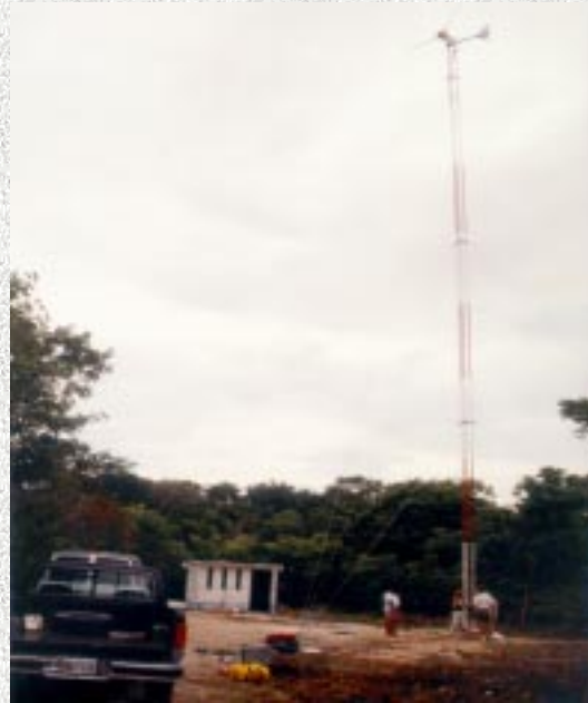
Pump house and turbine provide clean water in Quintana Roo, Mexico
