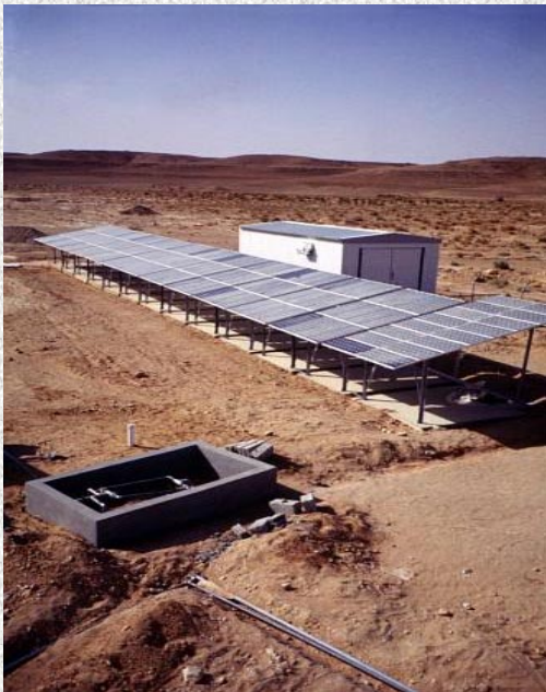
Wellhead, Panels, and RO Unit
