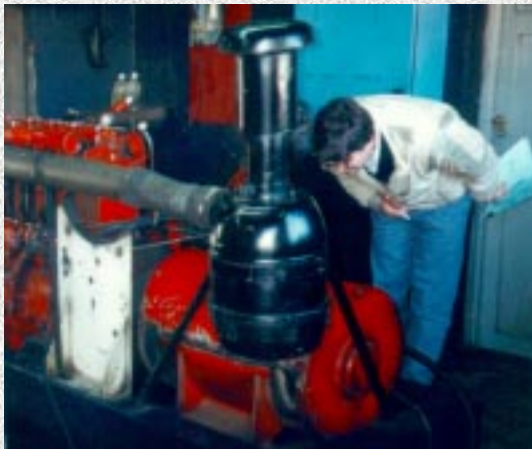
An isolated diesel plant in Tres Lagos, where a wind-diesel retrofit is under development
