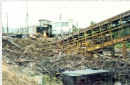
Site for a 1-MW Biomass Power Plant in Verkhne-Ozerski village, Arkhangelsk Region that will burn nearby wood waste.
