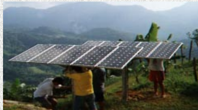
Panels installed by Solar Electric Company generate electricity to power a radio repeater station at the Regional Health Center of the Department of Health in Ormoc, Leyte
