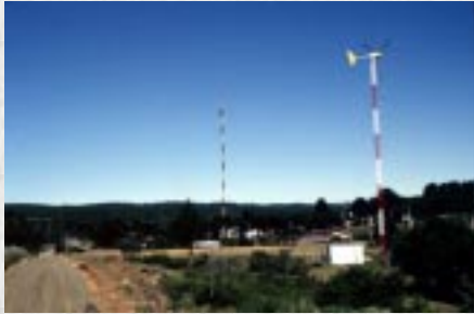
Village of Villa Las Araucarias and the installed power system
