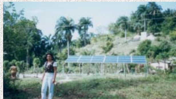
Typical ADESOL financed systems supply 2,000 gallons of water per day for 200 people
