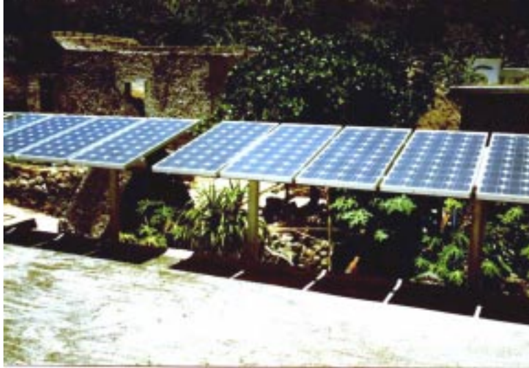
Figure 9 PV installation in Batanes
