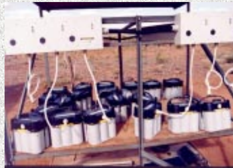
12 outlets with LED SOC indicators and batteries hvd protected
