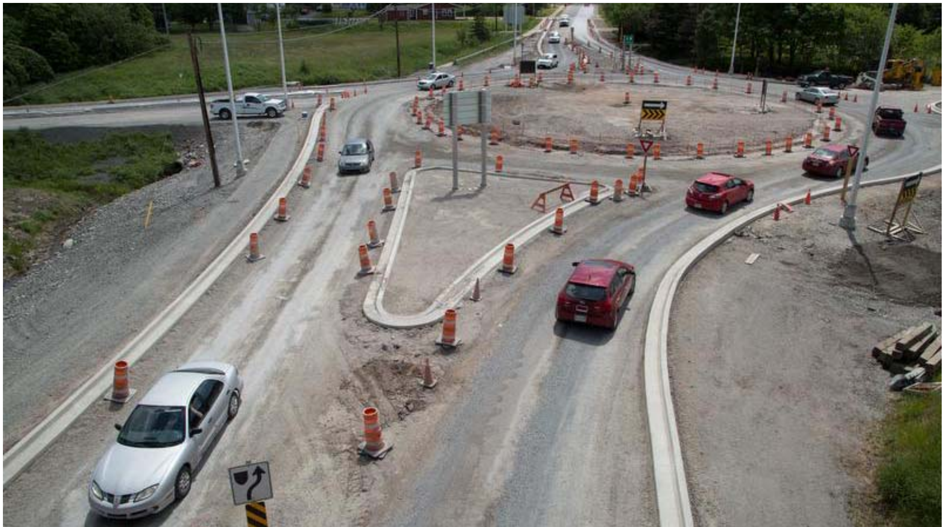
The George Street roundabout at Exit 8 off Highway 125, shown here July 2, is expected to be completed this summer. STEVE WADDEN
