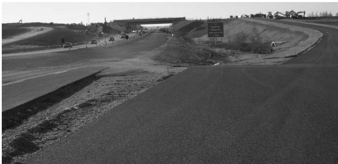
This latest project will leave the entire length of Highway 125 twinned when it’s completed, likely by next year. CONTRIBUTED/NSRBA
