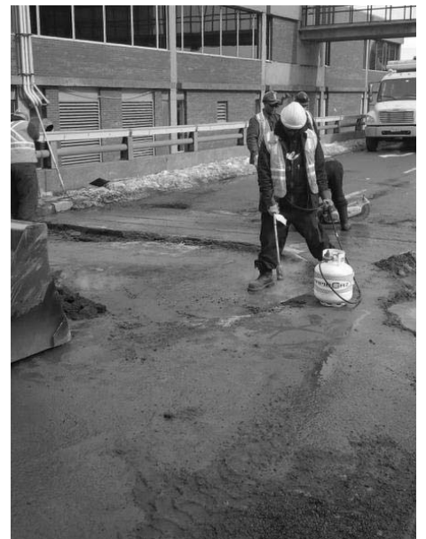
Weather and air temperature are big factors in proper pot-hole repair. CONTRIBUTED/NSRBA
