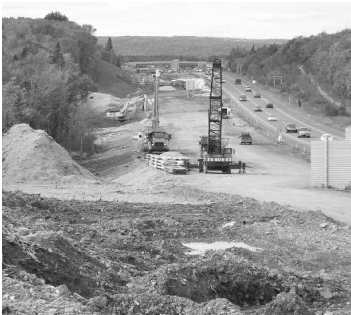
The Sydney Bi-Pass, as Highway 125 is sometimes referred to, takes commuters and travellers from Sydney Mines near the terminus of the Trans-Canada Highway to Grand Lake Road near Glace Bay — serving as the main transportation artery around the outskirts of Sydney as it traces its path around the city. CONTRIBUTED/NSRBA
