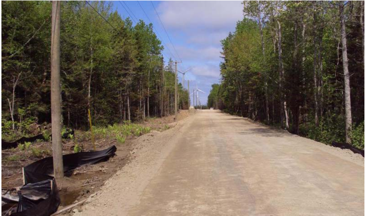
Nova Scotia's road builders have been meeting the challenges of building access roads required to build and maintain wind turbines. CONTRIBUTED/NSRBA
