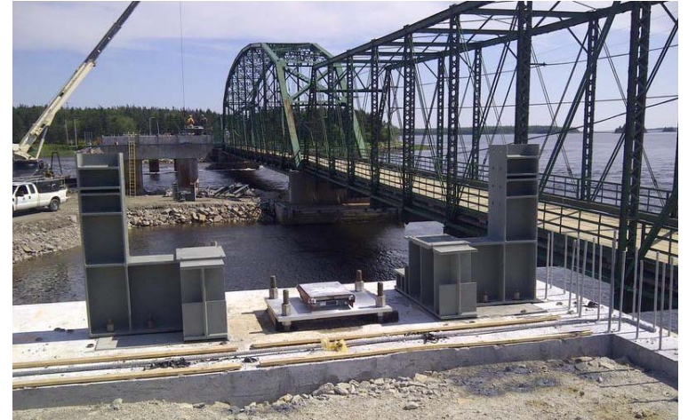
Indian Sluice is the channel between Sluice Point and Surette's Island in Yarmouth County. The existing bridge was installed in 1909. It will soon be replaced with a concrete, two-lane bridge. CONTRIBUTED/NSRBA
