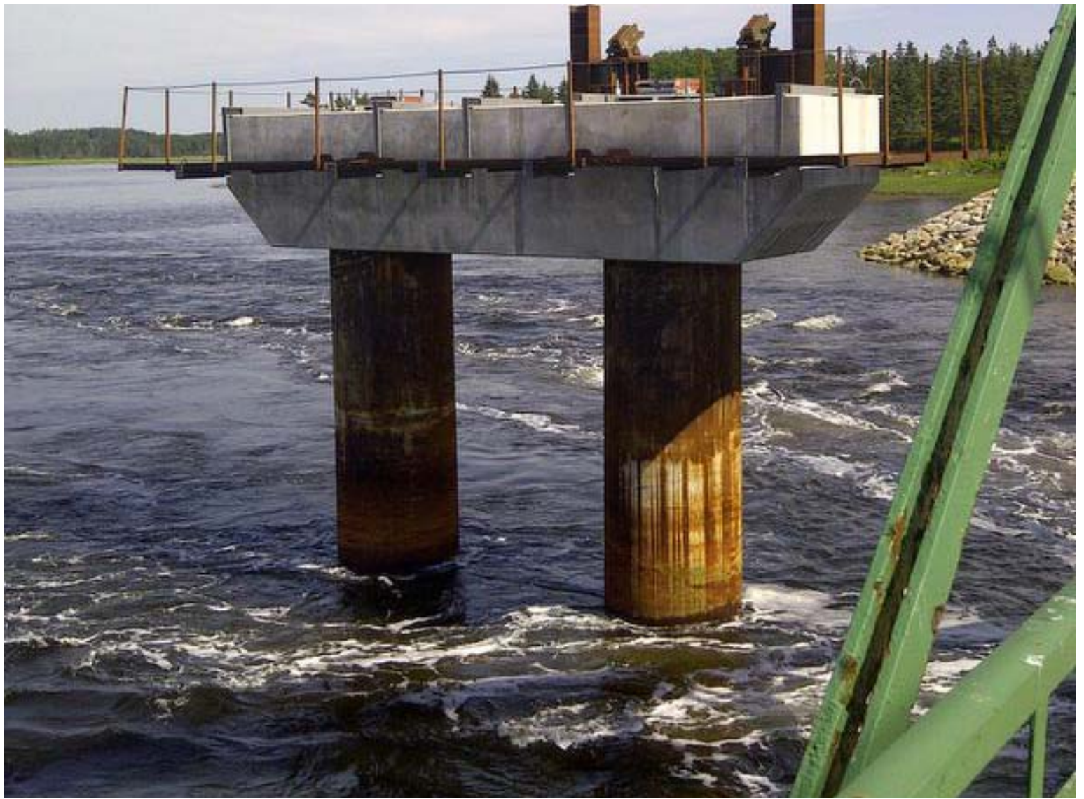
The Indian Sluice Bridge construction is one of several major projects underway right now in Nova Scotia. CONTRIBUTED/NSRBA
