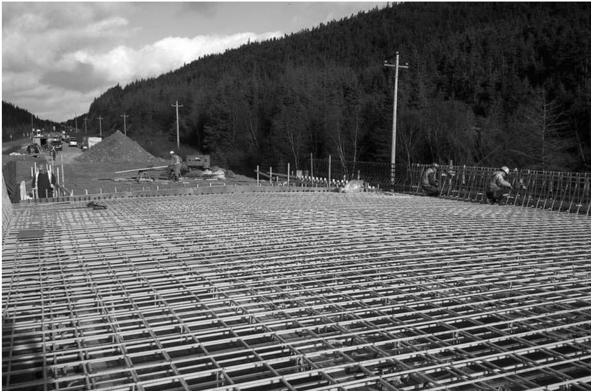
The Rattle Brook Bridge was built using the revolutionary, Nova-Scotia-invented glass fibre reinforced plastic mesh instead of the more traditional steel rebar. CONTRIBUTED/NSRBA
