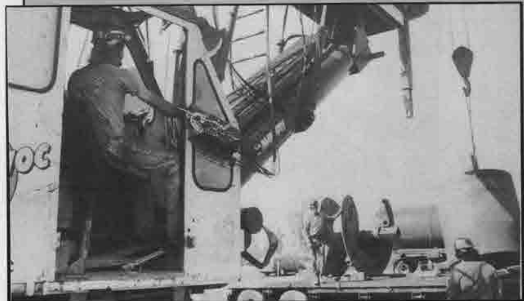
Below: Crane operator Randy Virdell of Muhaffey Drilling, a Benco subcontractor out of Southern California, uses a Manitowoc 2900 WC to lift pre-cast materials for bridge columns on Belmont Avenue.
