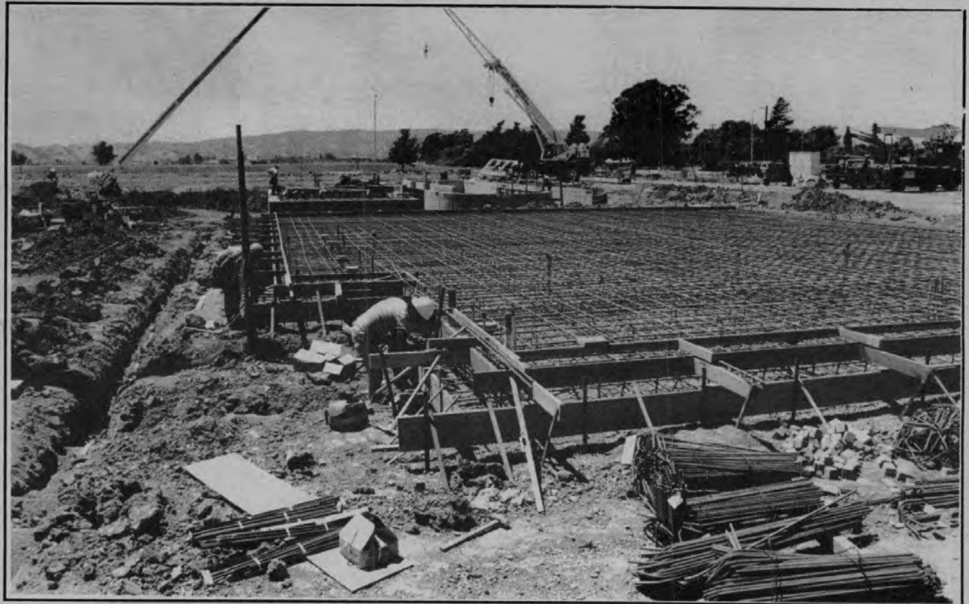
Kawah Construction (above) is currently working on a $14 million expansion of the Vacaville sewer treatment plant in Elmira. Operating loader on this job (lower left) is Jack Fullerton.
