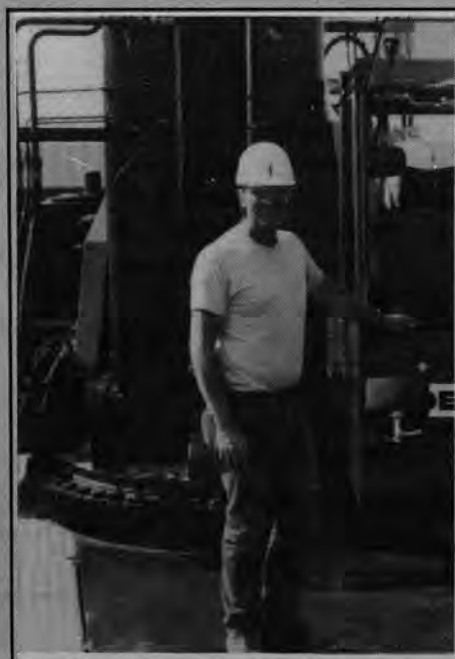
Pictured above is the Demag crane brought into Hill Field, Utah where OWL Construction is working on an MX missile silo. Pictured left is operator Ron Haagenen. Pictured below (left to right) are Ray Jessop, District Repr. Don Strate, Adrian Shippen and Ron Haagenen.
