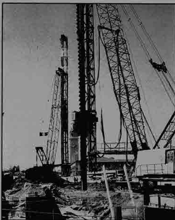
At times, the job site has looked like a forest of booms, drilling rigs and pile drivers. At one time in July, there were 13 cranes on the job.
