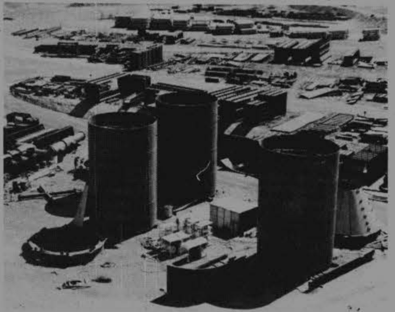
Portions of the combustion chambers waiting for assembly
