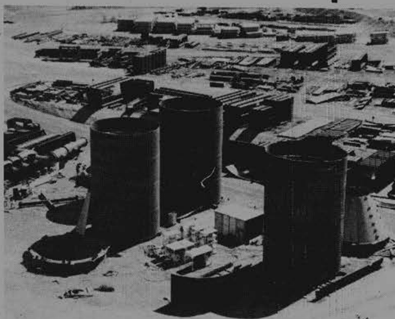
Portions of the combustion chambers waiting for assembly
