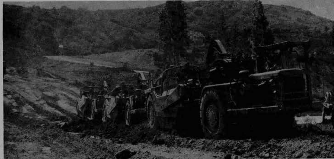
AS THE PICTURES ABOVE INDICATE, work is going full steam ahead on the modernization of Kaiser Permanente's Cement plant near Cupertino. Despite statistics showing that the new plant will reduce emissions by 52 percent in comparison with the current facility, Kaiser still met stiff opposition from environmentalists and town residents. Working the dozer in the top photograph is John Escover. Scraper operators are Elmo Riccio, Duey Davis, Lloyd Hack, Don Wise and Harold Batye. Other Local 3 members on the job, which is contracted out to "Buz" Haskins are Richard Smith, Jim McGee, Herb Meyers and H. P. Martin.
