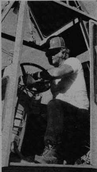
Don Malan (above) works hydraulic crane at PG&E's Geysers Units #15, while (right) Ron Lyons runs hydraulic lift on Unit #13.
