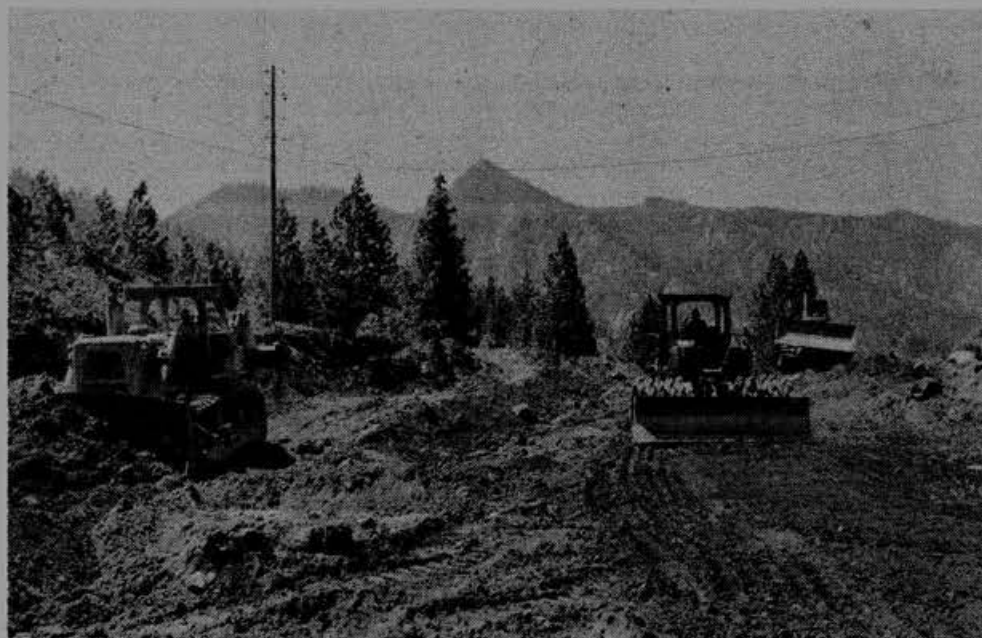
Photographs on this page were taken at the Markleeville Forest Service Road realignment project in the High Sierras. According to Stockton business rep. Bob Blagg, the $3.2 million project contracted to R.D. Watson will provide work for about 15 members throughout the summer.
