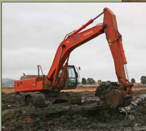
Henry Madrid operates an excavator in the mud at the Dutra Salt Pond project in Napa.
