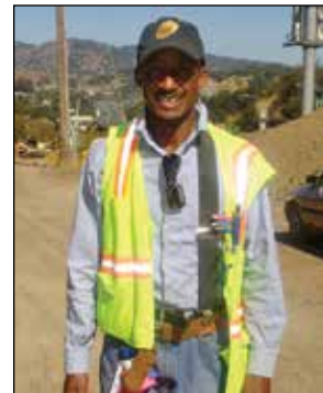
Member Dennis White checks grade for Ghilotti Bros., Inc. on Hwy. 101 in Marin.
