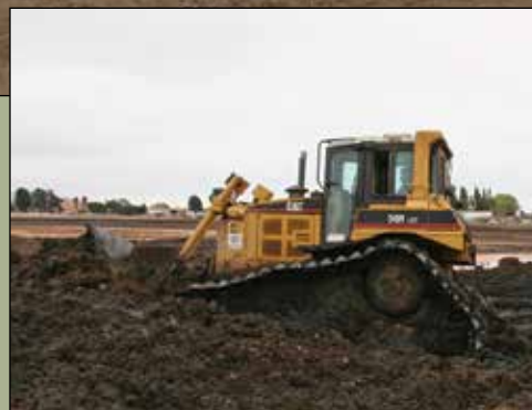
Albert Carabajal operates a dozer in the deep mud. The cable located on the back of his machine is used by other equipment to pull him out of the mud if and when he gets stuck.
