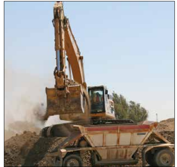
Excavator Operator Mike Gomes works for Asta Construction in the Fairfield District.
