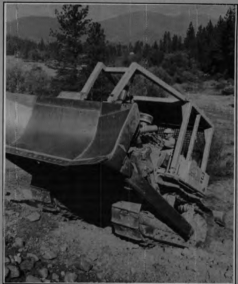
Local 3 Operating Engineers working on the Trinity Alps Business Park project are (top photo, from left): Jerry Shriner, a two-year member, D-8 dozer; George Erdahl, 25 years, D-8 dozer; Local 3 Business Rep. Wendell King; Louis Cannon, three years, TS 14; David Cellis, 10 years, TS 14; J. W. Brashear (owner), 28-year member; Steve Brummett, 18 years, TS 14; Superintendent Bruce Humphreys. In photo above: James Kane, 28 years, operating a D-6 on the Brashears project.
