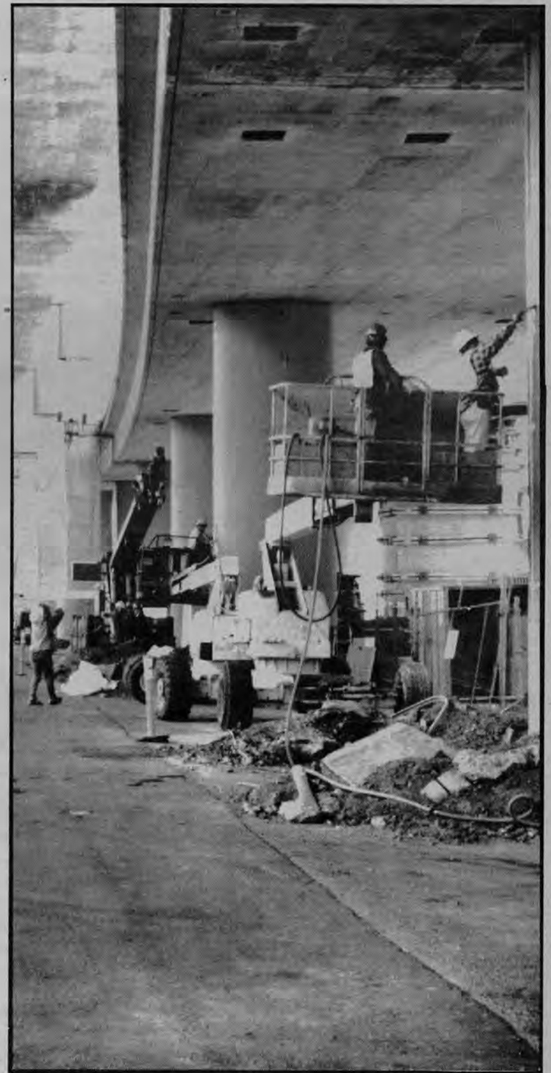
Operating Engineers and ironworkers were working on this section of the Southern Freeway viaduct before the project was shut down because of major design changes.
