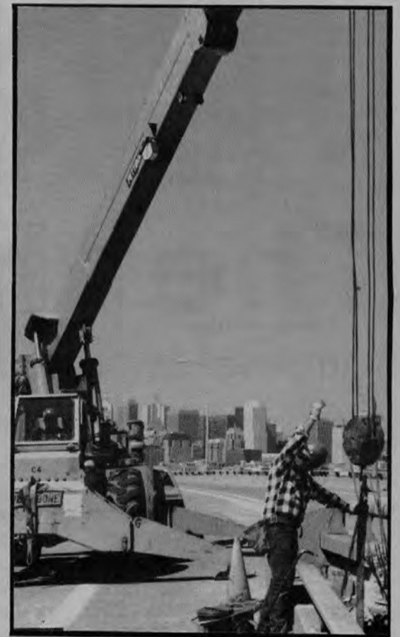
Above: Crane Operators working on the China Basin viaduct pulled cable restrainers into position.
