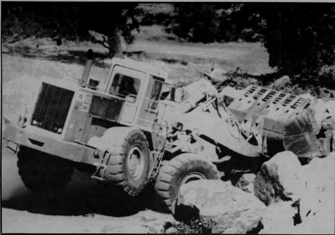
Rocks are stored adjacent to the highway right-of-way before being hauled to other projects for use as rip rock and rock slope protection.
