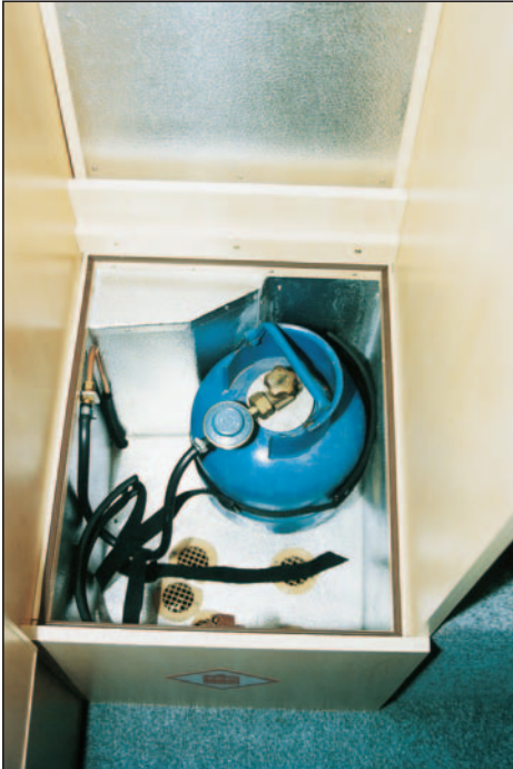
Beneath the wardrobe is the gas cylinder locker.
