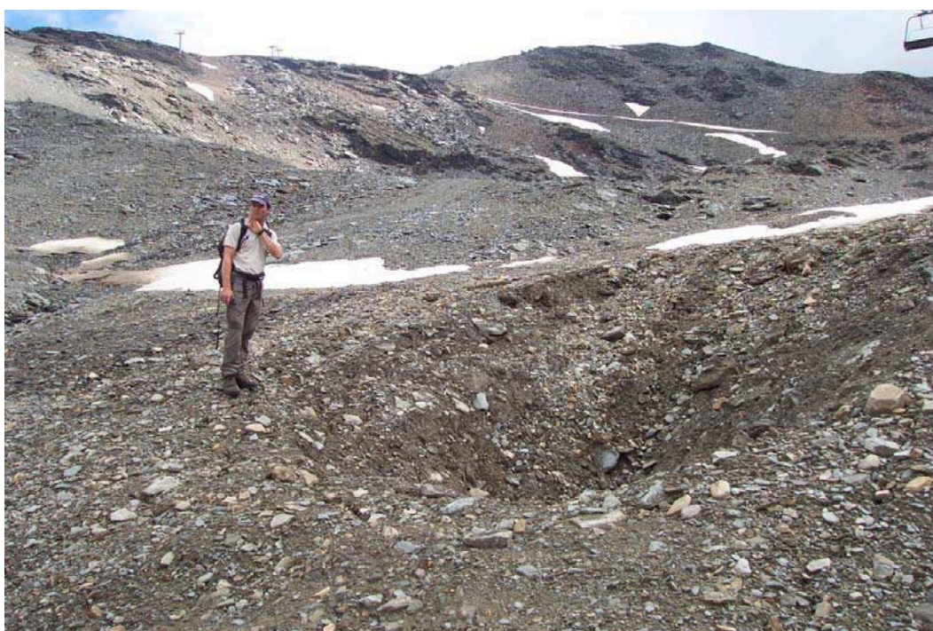
Fig. 7 – Photograph of subsidence processes in the vicinity of pillar no. 12 of the ski lift "Madritschjoch" in July 2006. Photograph by A. Zischg.
