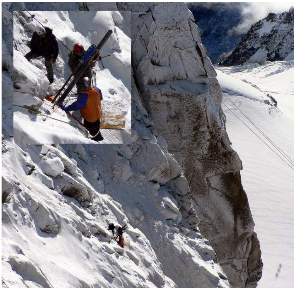
Fig. 3 – Drilling of a 10 m deep borehole in the southeast face of Piton central in September 2009. Photograph by P. Deline 17.09.2009
