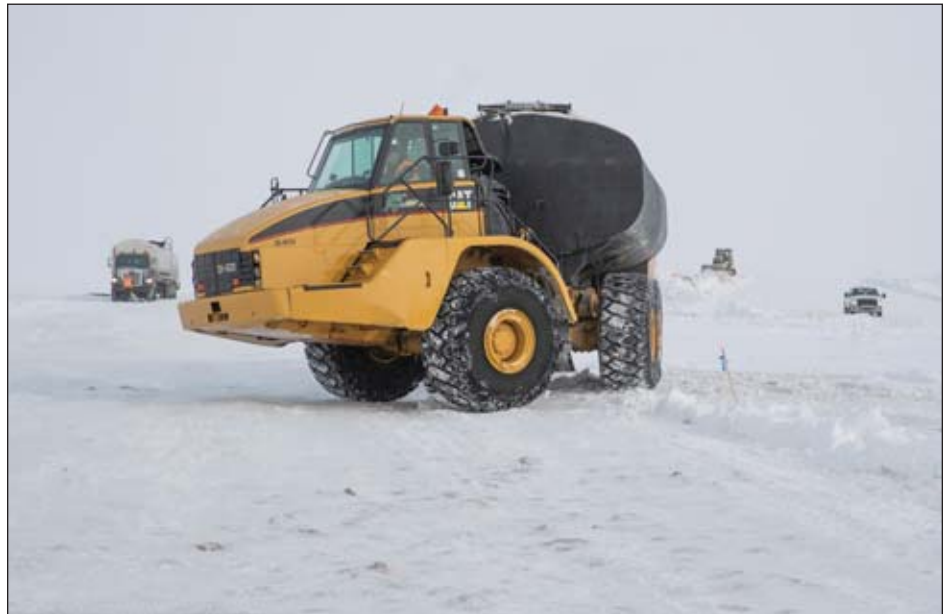
A truck lays ice chips for construction of an ice pad for the Willow project. April 2023.
