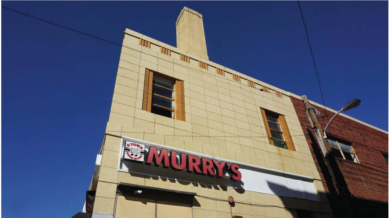
Figure 7 Detail of the terra-cotta cladding on the building's southeast façade. November 2019. Photo by Author.
