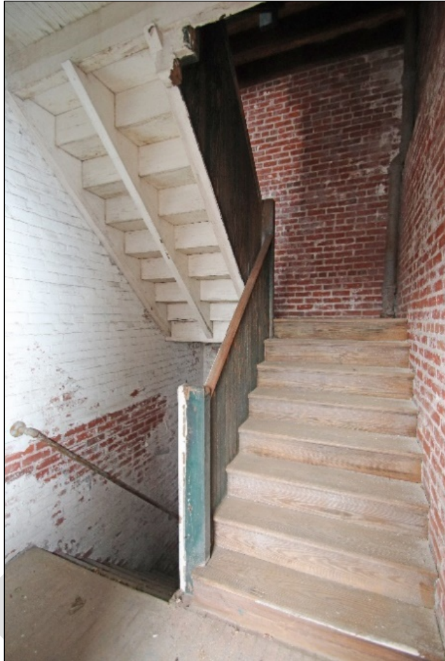
Photo 8 (right): U-return wood stair at the northeast corner of the building, looking west on the second floor.
