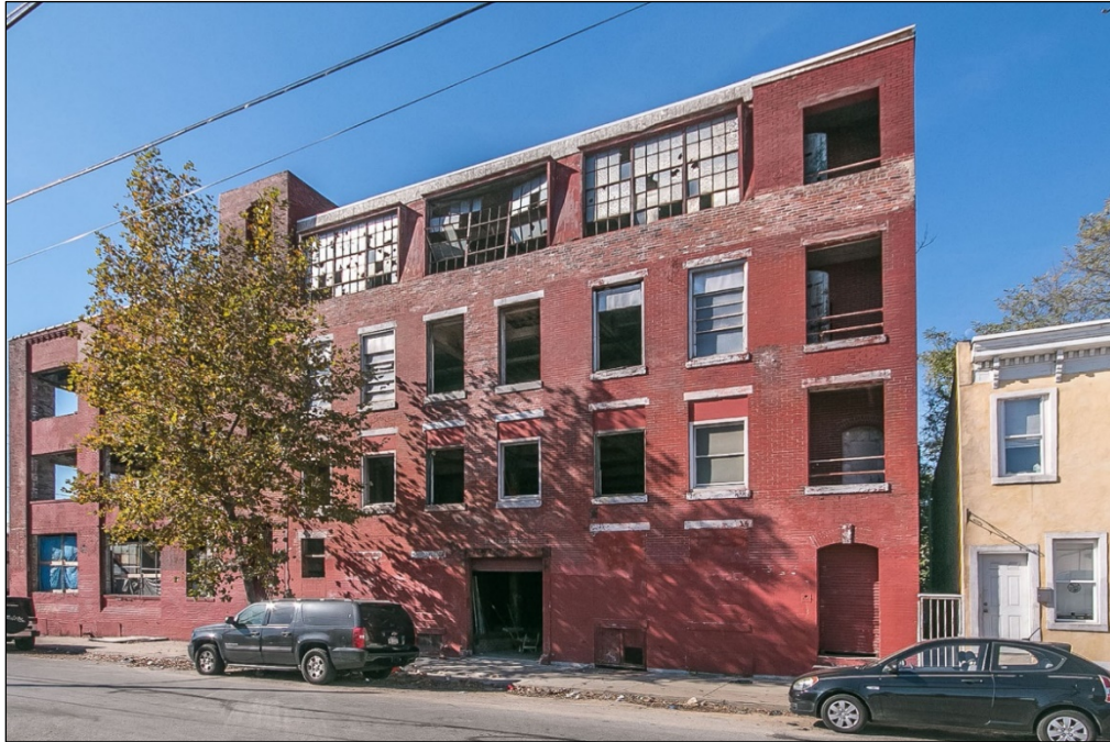
Figure 17: View of the building around 2020, prior to the removal of the windows
