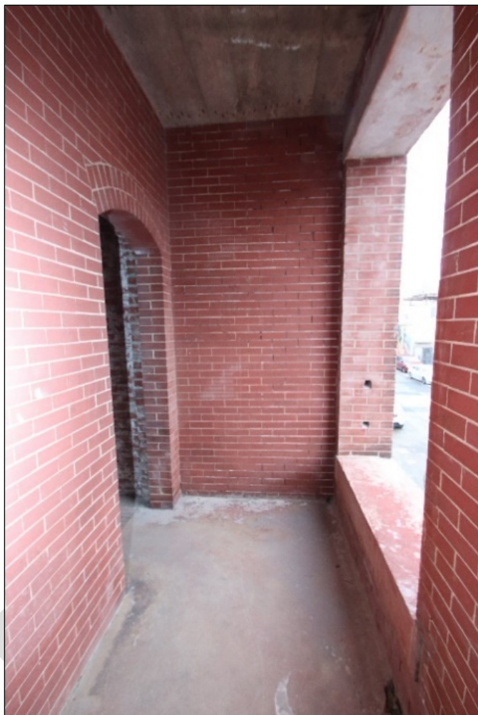
Photo 9: Typical fire balcony, located adjacent to the U-return stair at the northeast corner of the building, looking north on the second floor.
