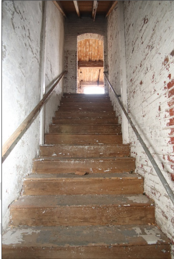
Photo 7 (left): Straight-run wood stair along the south wall, looking west on the first floor.
