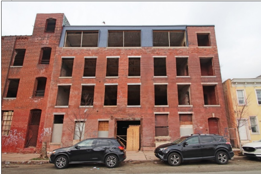
Photo 1: East elevation, looking west. The first four bays (from the left) on the first through third floors comprise the original circa 1870 building. The remaining three bays comprise the 1916 addition. The fourth-story mansard roof was added around 1924.
