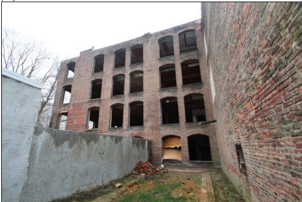
Photo 2: West elevation, looking east. This photo was taken from the vacant property at 1907 N. Marshall Street, which is not included within the proposed National Register Boundary.
