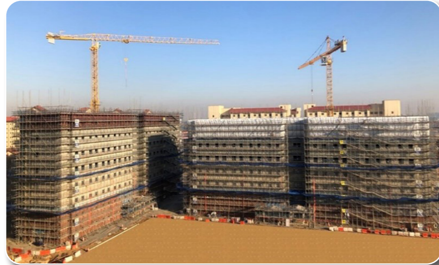
UEH120B Unaccompanied Enlisted Personnel Housing
