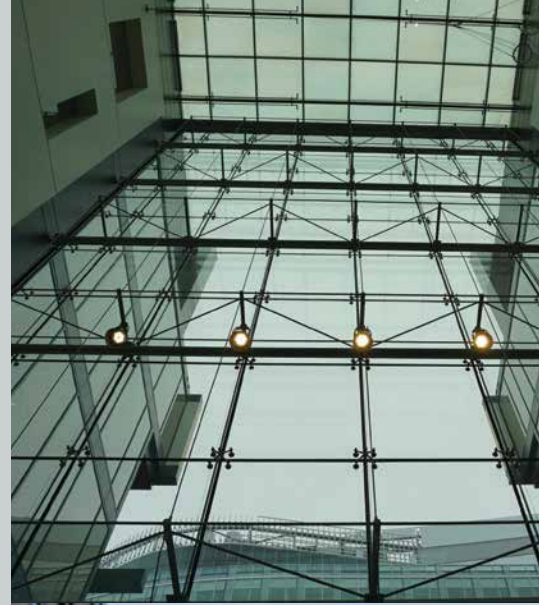
75-125 Binney Street - Alexandria Center, Boston, MA LoE 366 Structural Point Supported Insulating Glass Units Payette Associates ▶
