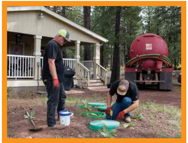
▶ Chase watches as technician Mike Bolen secures the riser lids after a pumping job.
