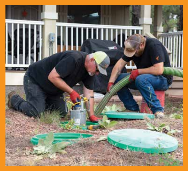
Chase inspects an onsite system utilizing a Norweco Singular aerator system, while Mike Bolen pumps the tank.
