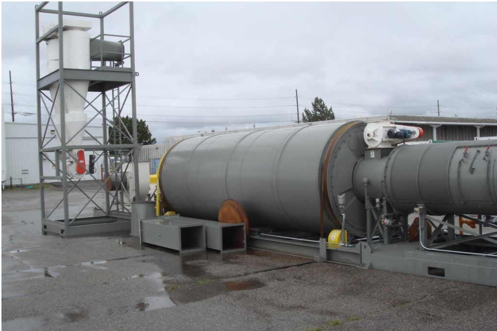
Figure 9. Rotary dryer used in biomass industry (Idaho National Laboratory (INL), 2016a) (Source: Biomass National User Facility, Idaho National Laboratory, Idaho Falls, ID).
