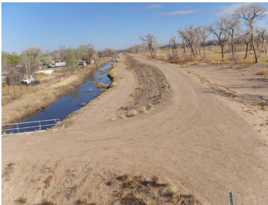
Figure 6.4 Riverside Drain, Dirt Maintenance Road, and the Engineered “Albuquerque West Levee” (Constructed in 2009), Looking North From the I-25 Bridge Over the Rio Grande. (A 2005 Fire Severely Damaged the Riparian Vegetation East of the Levee.)
