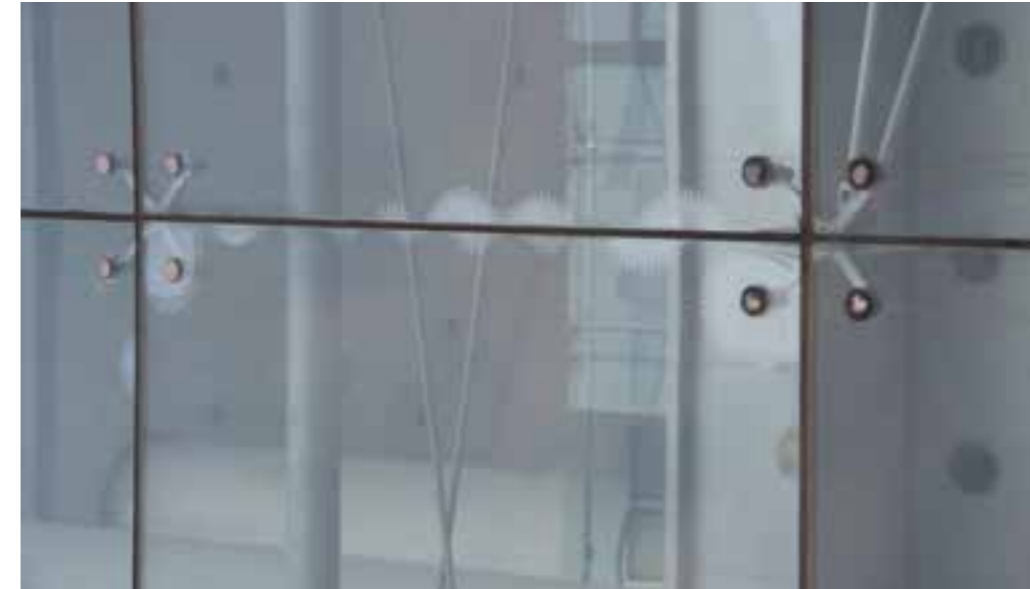
Typical defects caused by delamination.
