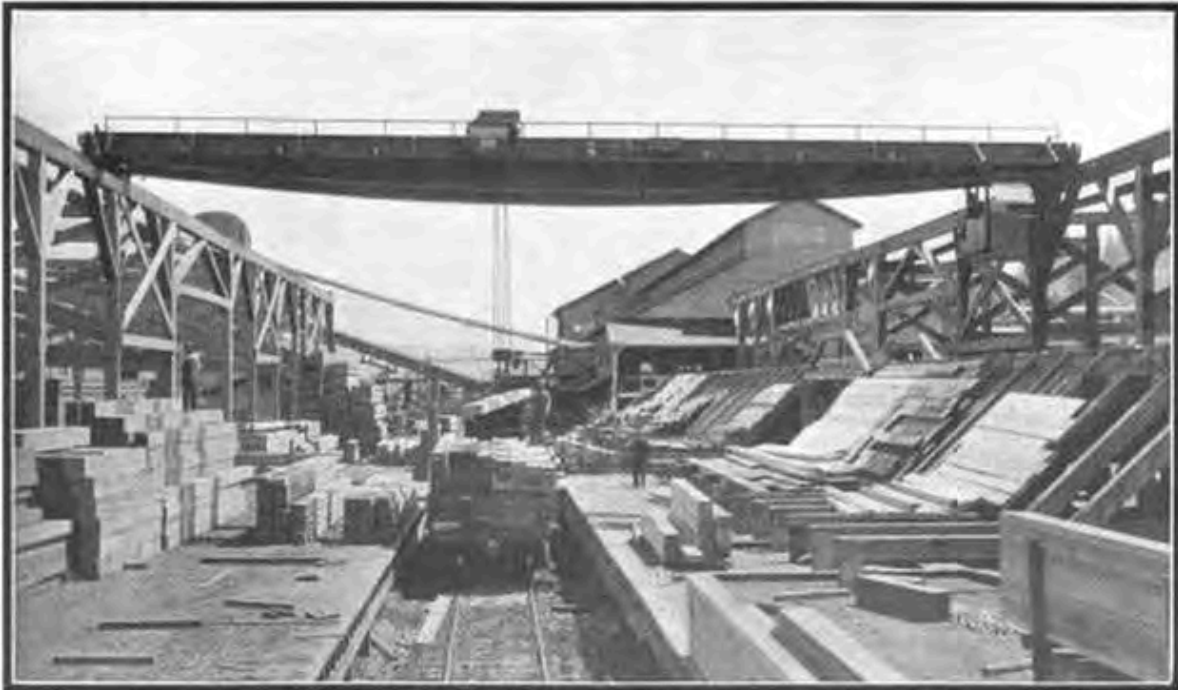
Pawling & Harnischfeger Crane recently installed at Booth-Kelly Lumber Co., Springfield, Ore., for handling heavy timbers
