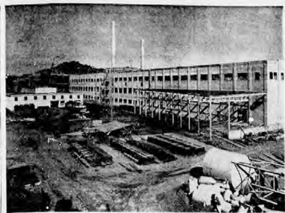
CONSTRUCTION at the Weyerhaeuser Timber Co plant in Springfield continues rain or shine and most buildings are close to completion. The machine room of the kraft pulp mill unit is shown here. The daily output of 150 tons of kraft pulp will be processed into container board. The kraft mill will utilize leftover sawmill slabs, edgings and trimmings, thus eliminating waste on the plant site. Low white building on the left is shop and warehouse for pulp mill. (Wiltshire engraving).
