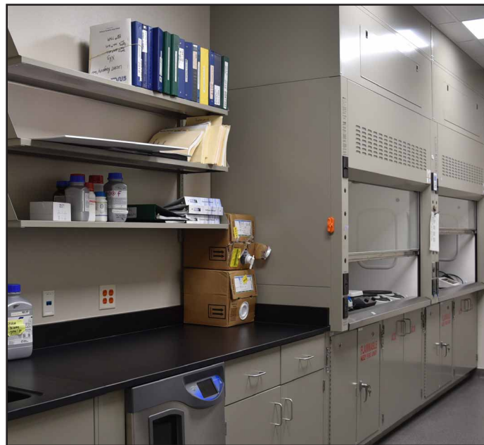
New Laboratory Fume Hoods
