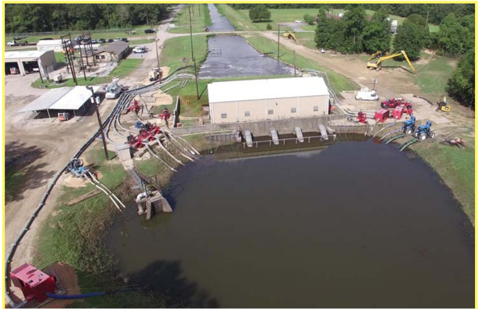
Temporary Pump Operations, Hurricane Harvey Flood Recovery
