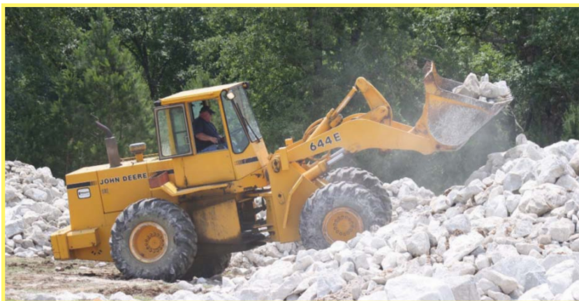
Shoreline Hardening Rip-Rap
