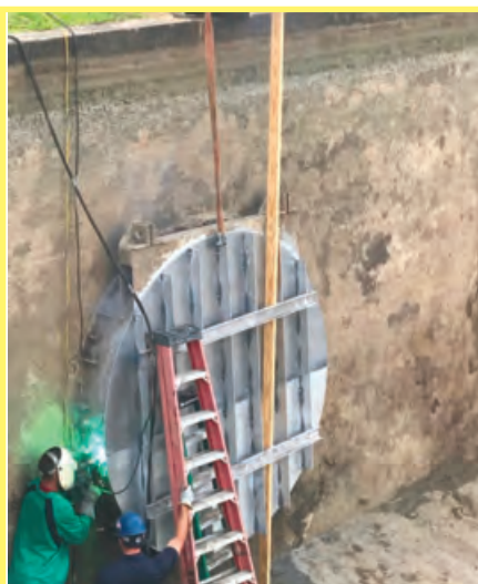
Sealed Pump #4 Flap Valve
