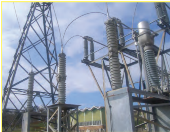
FERC-Regulated Toledo Bend Powerhouse
