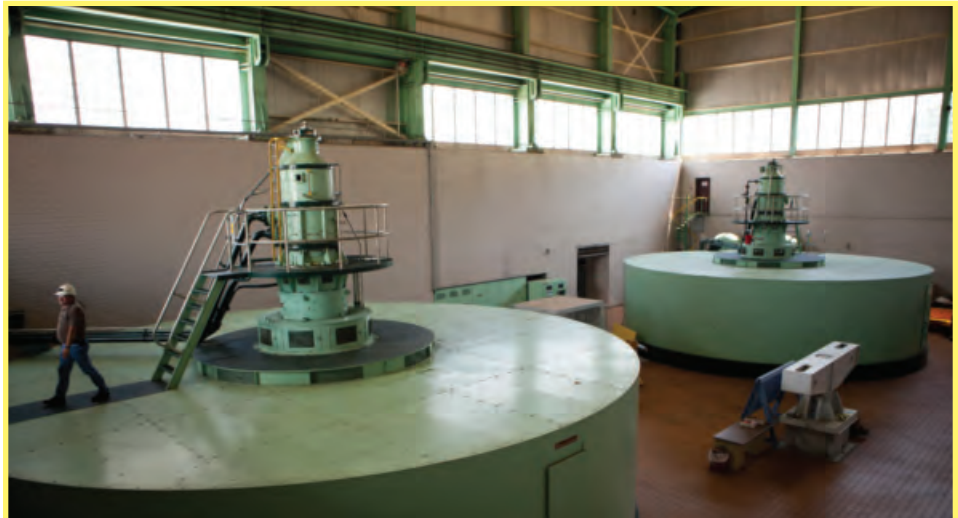
Toledo Bend Hydroelectric Generating Units
