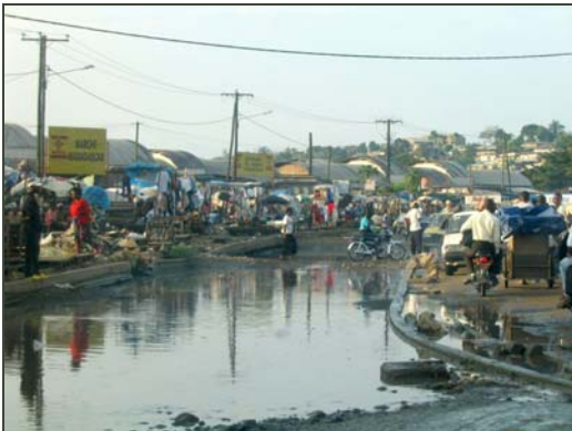
Road Failure at major junction
