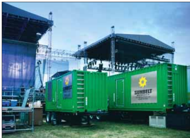
Cummins 500 and 1,000 kW Industrial Generators Power provided for an outdoor event
