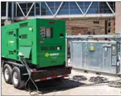
5,000 CFM Electric Desiccant Dehumidifier & 175 kW Generator
