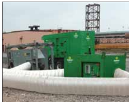
5,000 CFM Desiccant Dehumidifier, 320 kW Generator & 150 kW Heater
