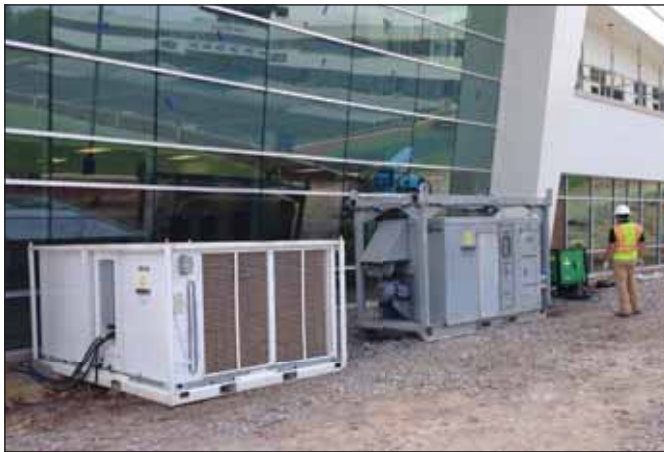
MobileCool MOB-250 25-ton Industrial Air Conditioner Temporary cooling application at a job site
