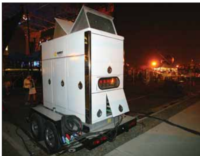
Crawford 1,400 amp Movie Set Generator Powering sound stages at an outdoor concert
