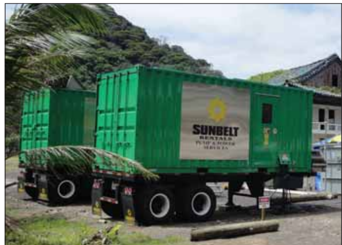
Two paralleled MQ Power 500 kW Generator Emergency power for disaster relief
