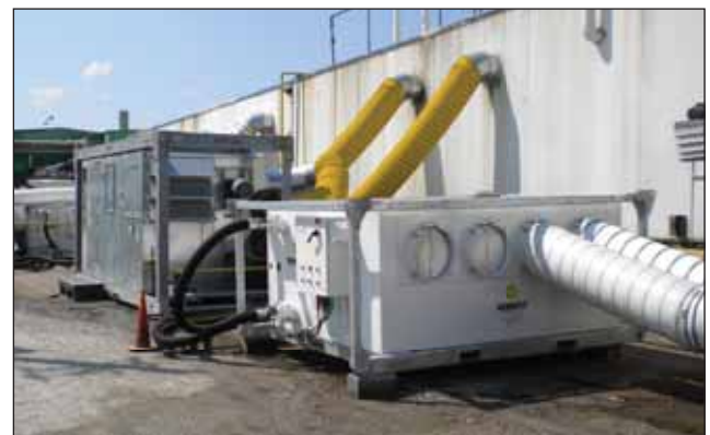
Desiccant dehumidifier and air handler at a processing plant
