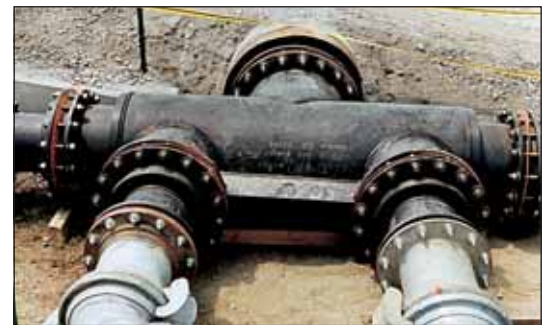
A 24" diameter HDPE manifold combining the flows of (4) 12" discharge lines on a sewer bypass project
