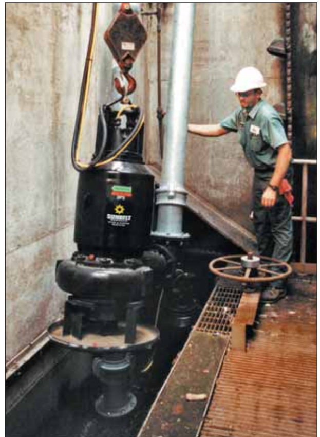
Gorman-Rupp 8" 70 HP Trash Pump One of four 8" trash pumps utilized on a wastewater treatment plant bypass job being lowered into a wet well
