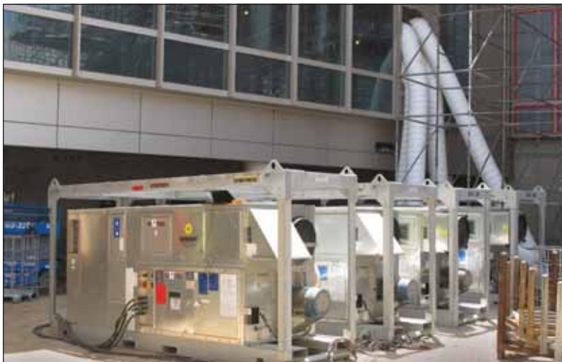
Above: Four 5,000 CFM Electric Desiccant Dehumidifiers in operation at a construction project in CA.
