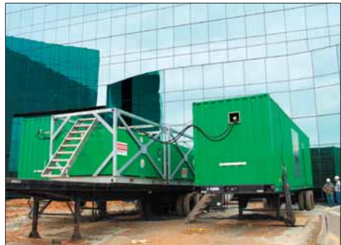
Two paralleled 1,500 kW generators and two 2,300 gallon auxiliary fuel tanks providing temporary power at a medical research facility
