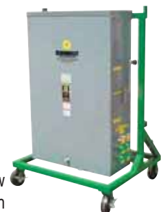
600A Double Throw Transfer Switch
