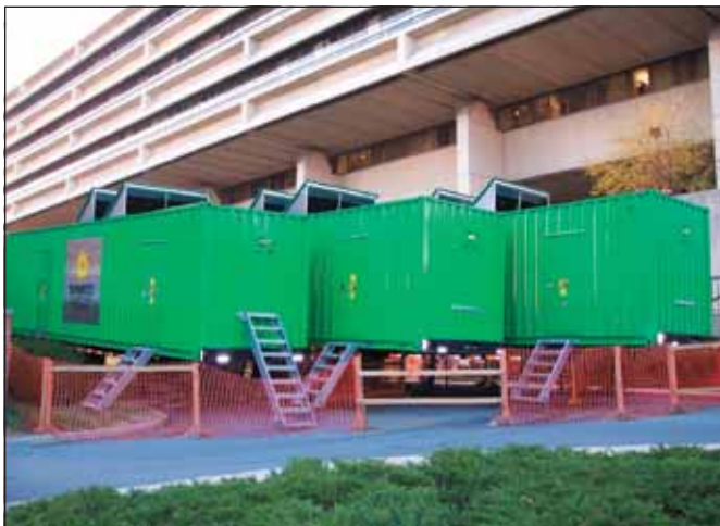
Three paralleled 1,500 kW generators providing emergency power at a military hospital
