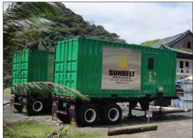
Two parallelled MQ Power 500 kW Generator Emergency power for disaster relief
