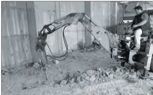
David Canini breaks rock on the ground level of the Museum's head office building during trench digging to lay sewer pipes.
