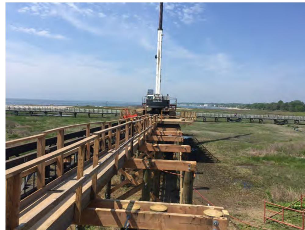
“Leap Frog” Method of Construction at Silver Sands State Park, Milford, CT
