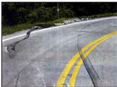
Figure 3.7 – These tire marks indicate that the vehicle's wheels left the road surface.
