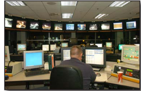
Figure 6.1 – Traffic control centers have myriad equipment used to monitor traffic and road conditions. (Photo/Bob Esposito, Pennsburg, Pennsylvania)
