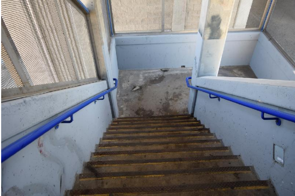
Image 6 (stairway does not appear to be subjected to regular steam cleaning)
