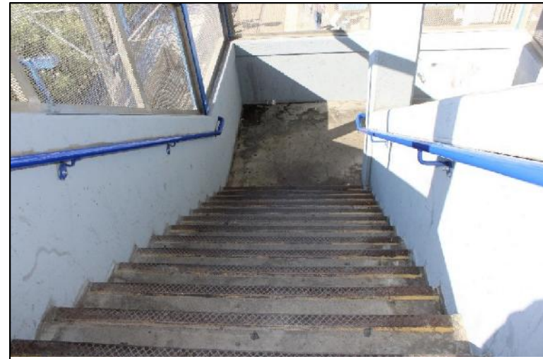
Steep, dirty stairs create an unwelcoming and unpleasant transfer environment.
