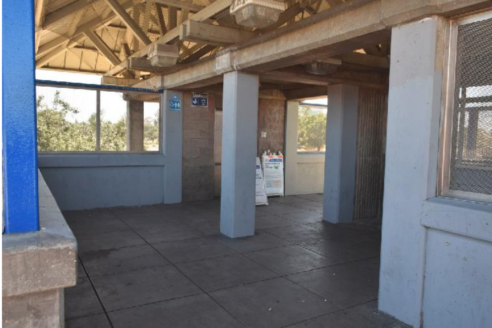
Image 2 (trash on ground, stains, dirty overhead, multiple barricade signs)
