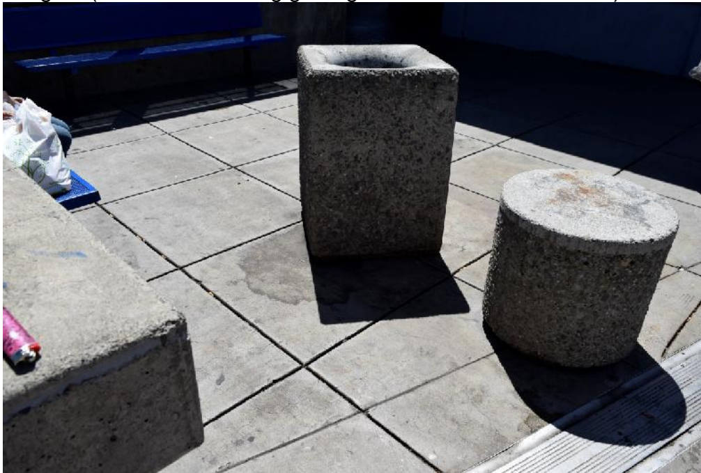
Image 3 (stains from leaking garbage can and on circular seat)
