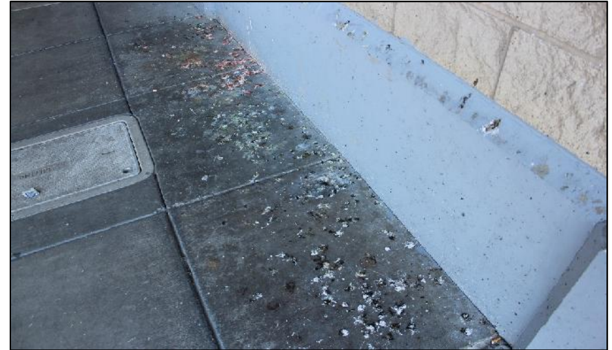
Accumulation of bird droppings.
