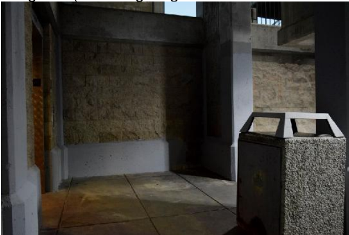
Image 15 (lack of lighting creates shadowed areas)
