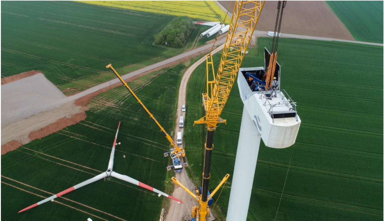
Dismantling wind turbines in Adorf am Diemelsee for ABO Wind. They will be replaced by two new, more powerful turbines at a later stage. The new turbines have three times the output of the old ones. Photo: Hagedorn
