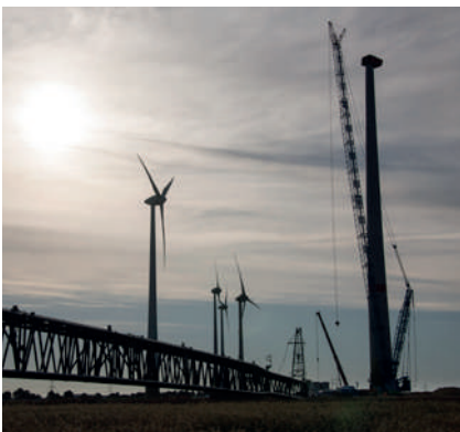
Heubusch wind farm near Meerhof. Photo: Ulrich Mertens
