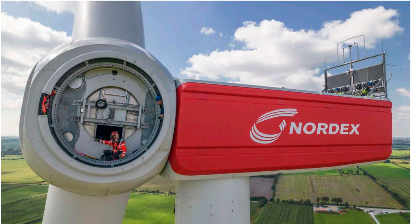
Fitting the third rotor blade on Prototype 1 of the N163/5.X on the test site at Janneby citizens' wind farm. Photo: Ulrich Mertens
