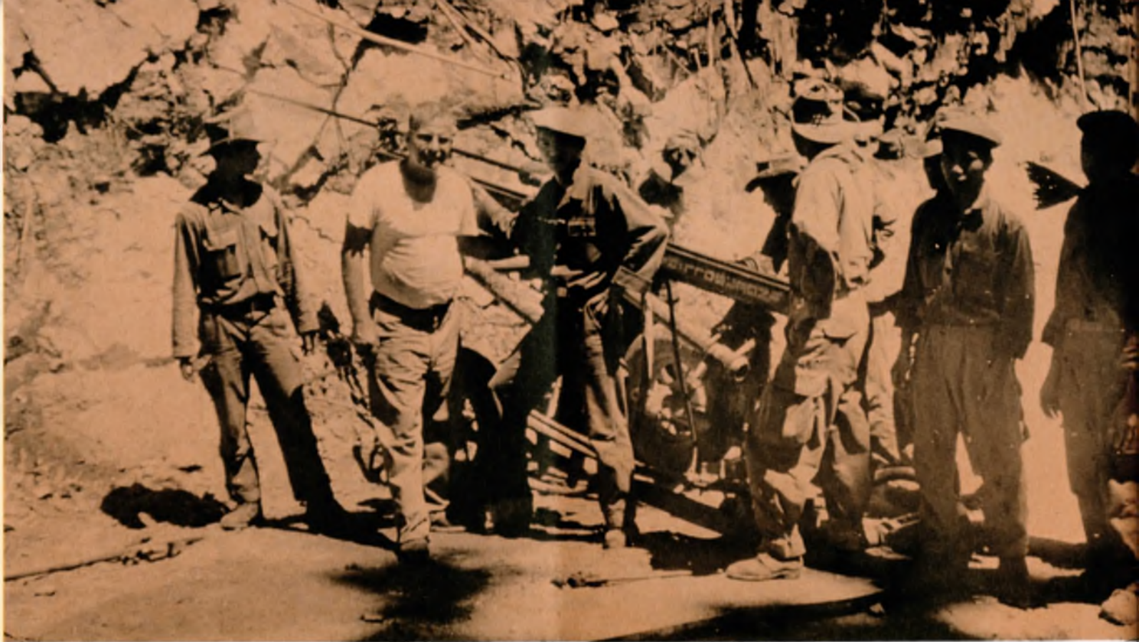
Philco TechRep Paul Bingeman instructs his Vietnamese crew in the operation of a rock drill preparatory to setting charges and blasting. Bingeman is part of a TechRep team giving practical instruction to native personnel building a highway across the rugged Viet Nam terrain.
