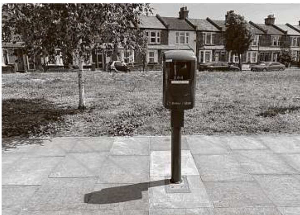
Newham in eastern London in June installed a pair of EV chargers partly funded by Uber.
