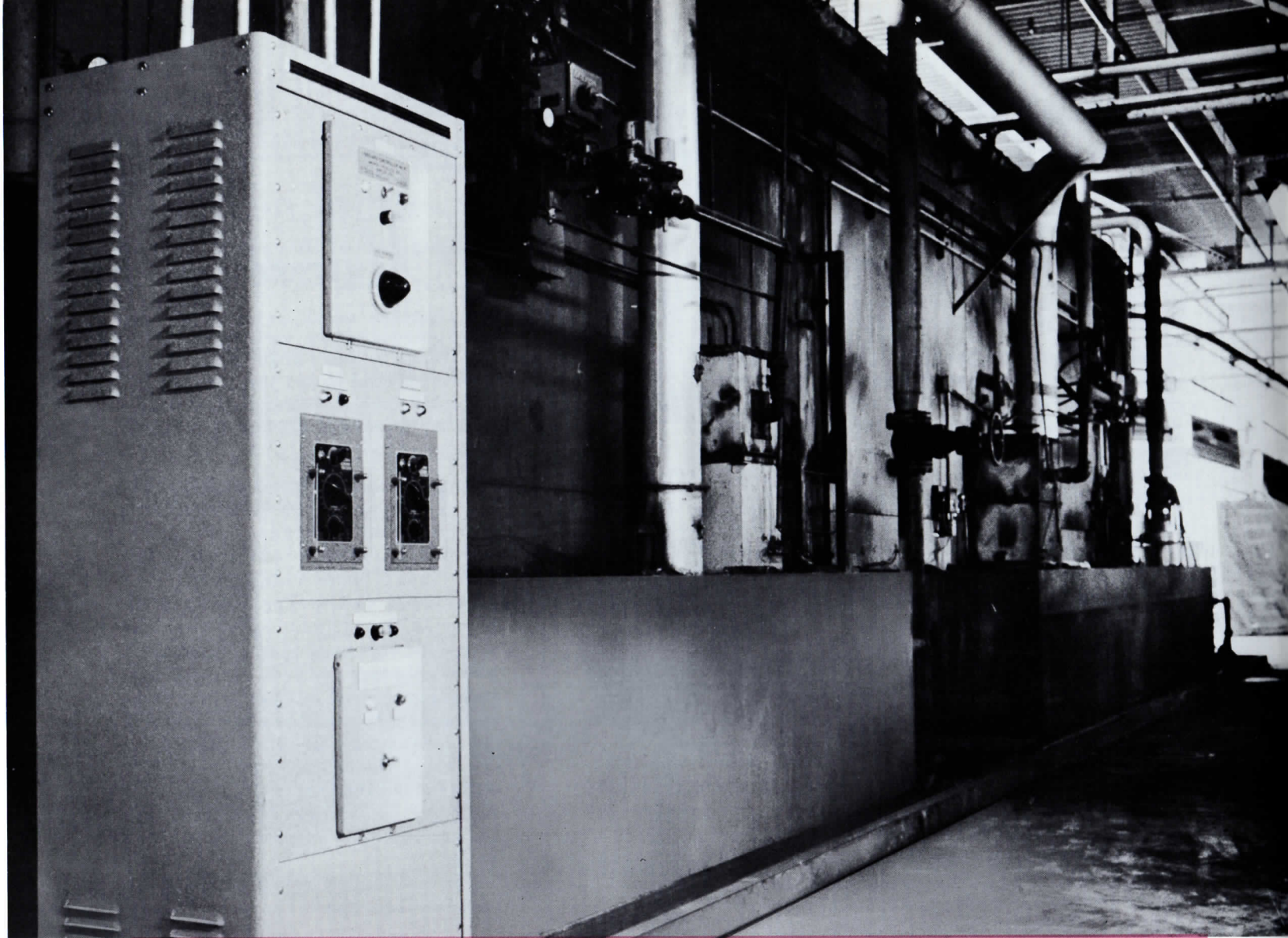
Part of the line for the pre-point zinc phosphate treatment process at Export Processing Corp., Detroit. View in foreground shows console for the new complete, automatic electronic control system developed by Amchem. The new process has six basic stages. First is the cleaning stage, second and third are rinsing stages, fourth is the coating stage, the fifth stage—rinse; the sixth stage—final passivating rinse.
