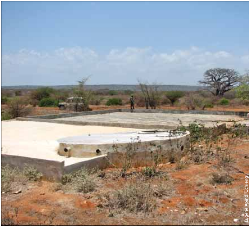
This concrete slab in northeastern Kenya collects rainfall and diverts it into an underground storage tank for later use
