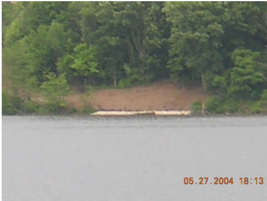
Lake Vermilion Bank Erosion
