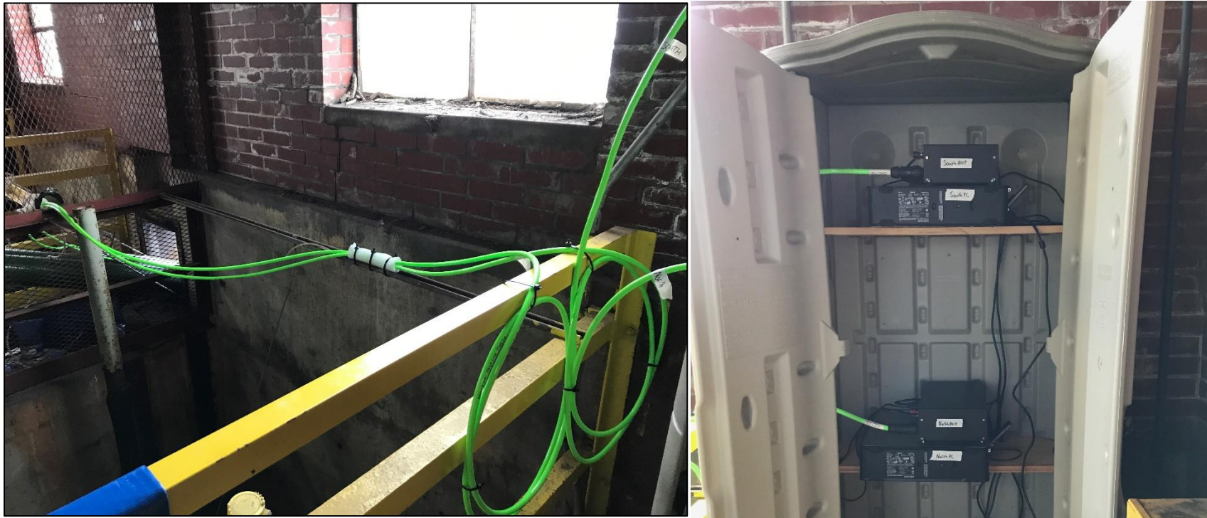
Figure C-2. Photos of the ADCP power and communication cable assemblies and the computer interface systems for the ADCPs, installed in Screen House #1 at Schiller Station.
