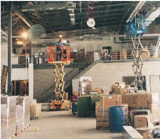
Construction of the Combined Services Building is progressing at the intersection of the Airport's main runways.
